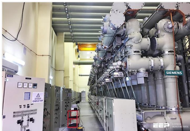
Figure 6.1. Gas Insulated Sub-Station and Grounding Area with Gravel Surface
