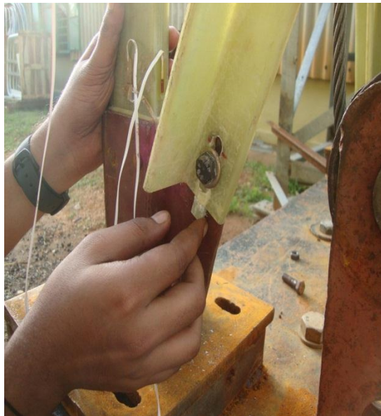
Fig. 4.18b Photograph showing failure of bracing member at bolt hole( TS2CA)
