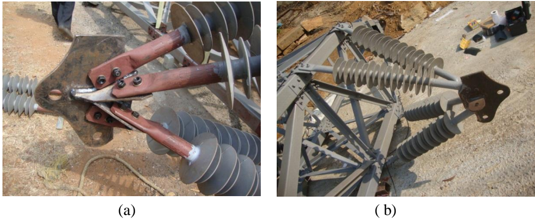
Fig 3.29 Photographs showing details of (a) connection at the tip of cross assembly and (b) Connections at base portion of the cross arm
