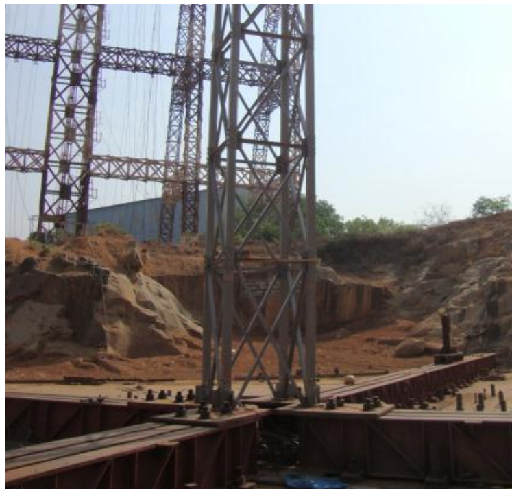
Fig. 3.31 Photograph showing tower mounted on rigid footings in testing station
