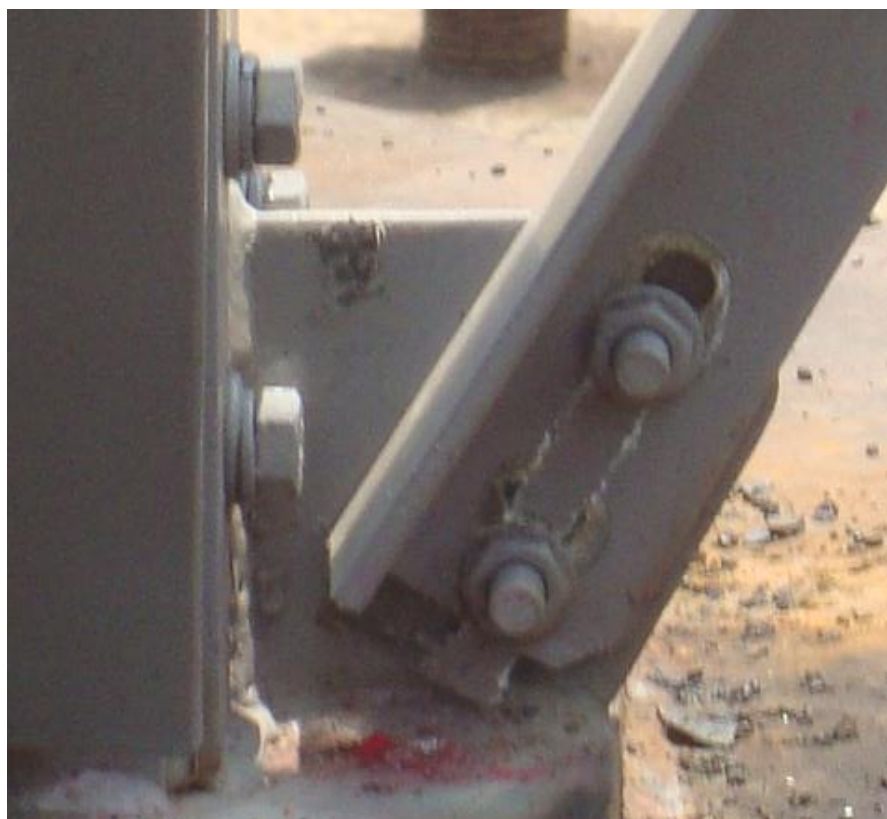
Fig. 4.22b Bolt sheared off at the joint between leg and bracing
