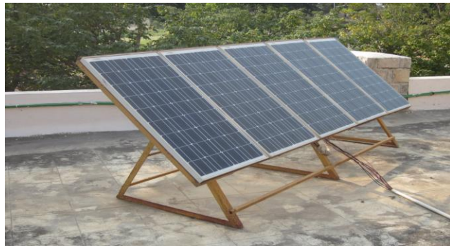
Fig.4.12 Solar PV panels used for experimentation.
