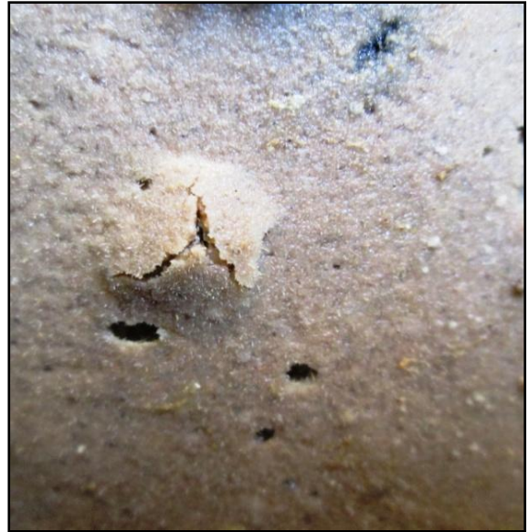
(b) Pop-out on the surface due to internal pressure exerted by aggregates
