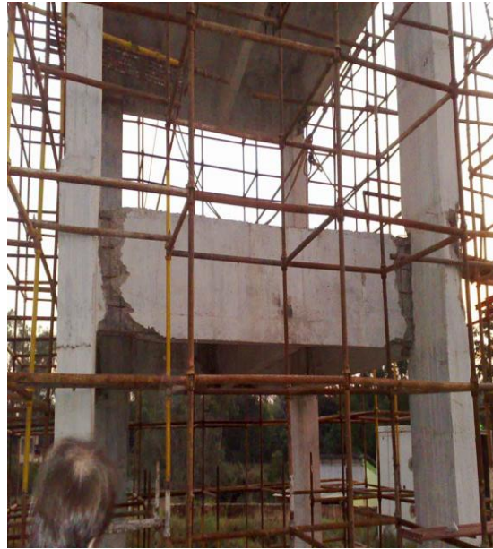
Fig 3.20 Torsional failure of Beam BF 225 after removal of loose concrete
