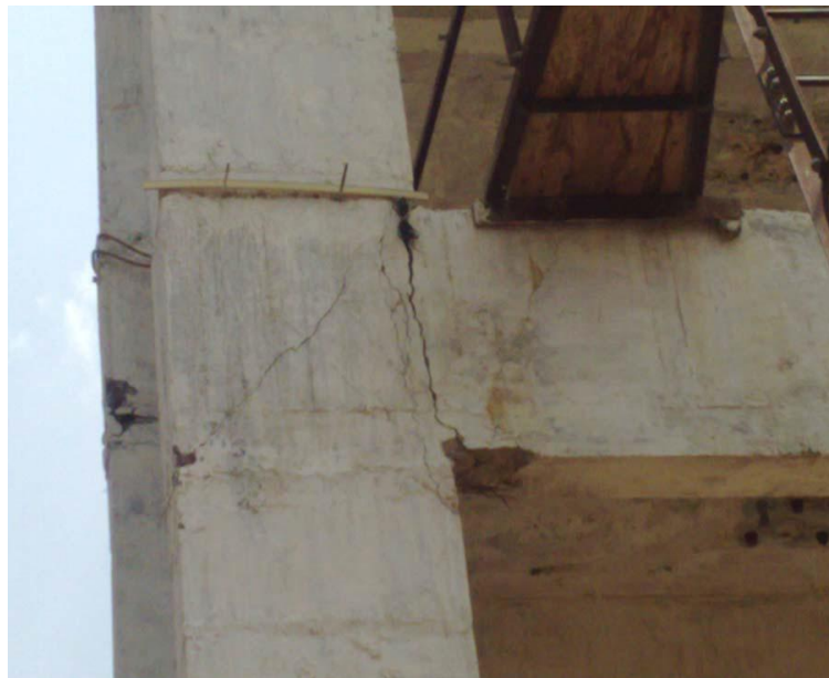
Fig 3.24 Joint failure of CL 16 due to bond at 2 nd floor level
