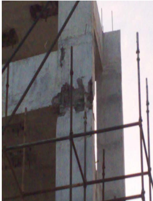
Fig 3.26 State of Joint of CL 20 at 2nd floor after removal of loose concrete
