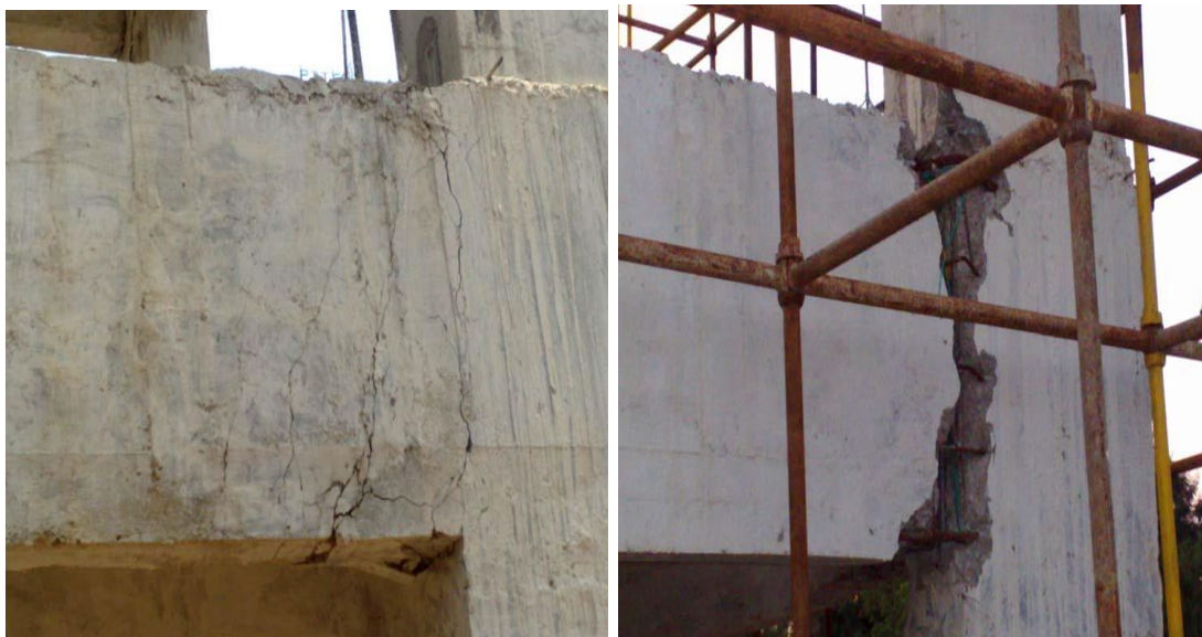
Fig 3.17 Failure mode of Beam BF 205 Fig 3.18 Failure mode of Beam BF 205
