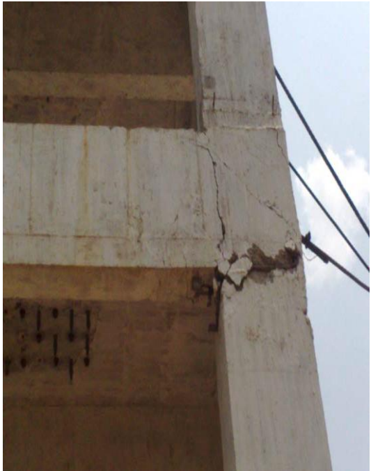
Fig 3.25 Joint failure of CL 20 due to joint shear, beam flexure and bond at 2nd floor
