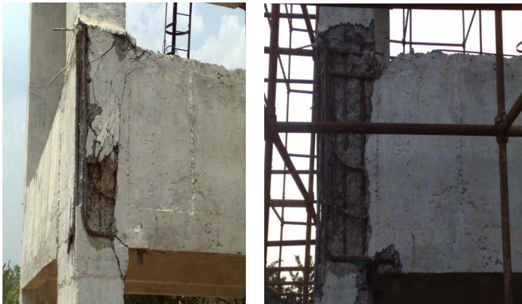
Fig 3.21 (a) Joint failure of CL 19 at 1 st floor during the test (b) State of Joint of CL 19 at 1 st floor after removal of loose concrete
