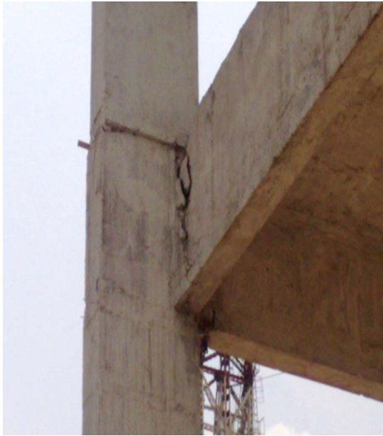
Fig 3.19 Torsional failure of Beam BF 225 while testing
