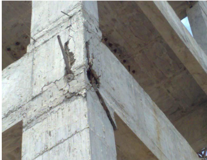
Fig 3.22 State of Joint of CL 19 at 2 nd floor after removal of loose concrete
