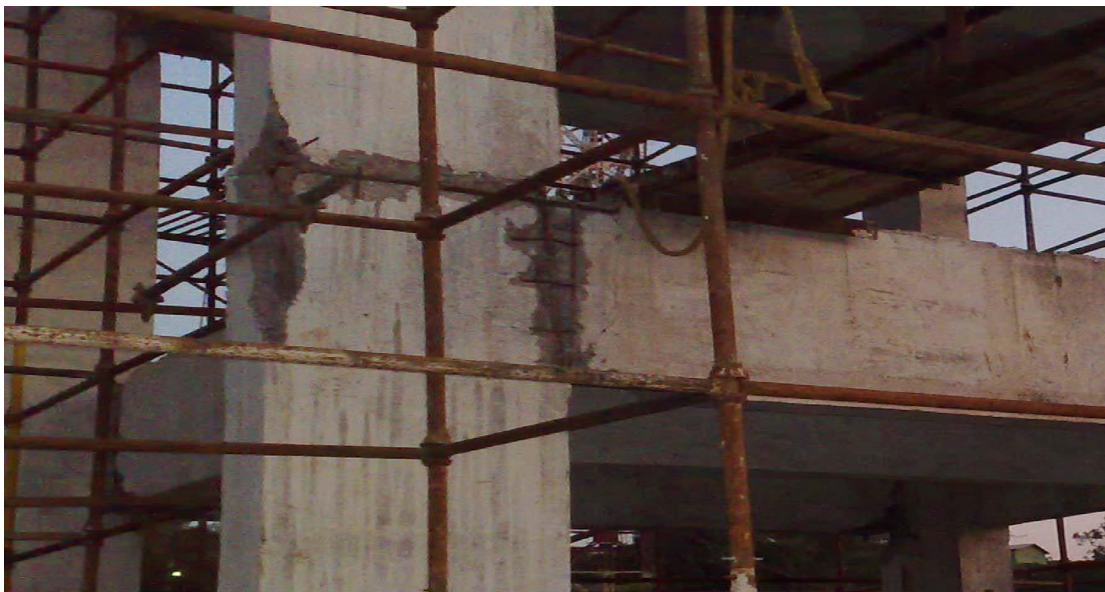
Fig 3.23 Joint failure of CL 16 due to bond at 1 st floor level
