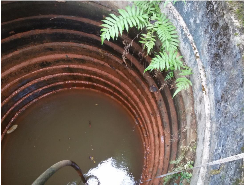
Fig.3.6 Photograph of pumping well no PW2
