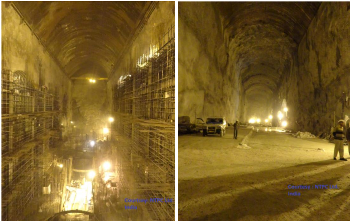
Fig. 2.4 Powerhouse and transformer hall caverns of Tapovan Vishnugad hydroelectric project, Uttarakhand (NTPC Ltd.)
