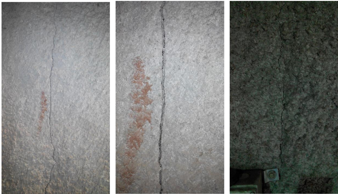
Fig. 4.68 Tension cracks on walls of bus ducts
